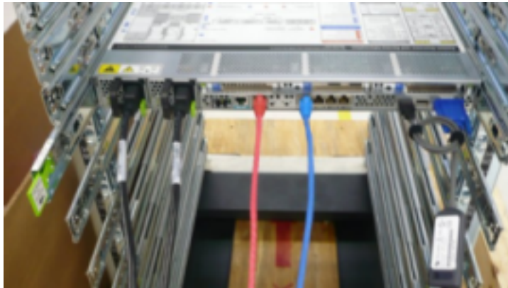
Figure 2-3 Cables at the Rear of the Server
