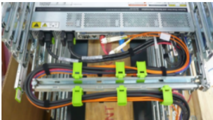
Figure 2-9 RDMA Network Fabric or TwinAx Cables Secured with Hook and Loop Straps at Regular Intervals
