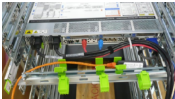
Figure 2-5 Cables Routed Through the Cable Management Arm
