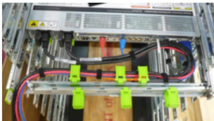
Figure 2-6 Cables Secured under the Cable Clasps
